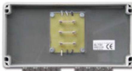
Diag.: Voltage transformer without cover with fuses
